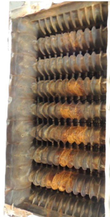
Multiple sections fractured
