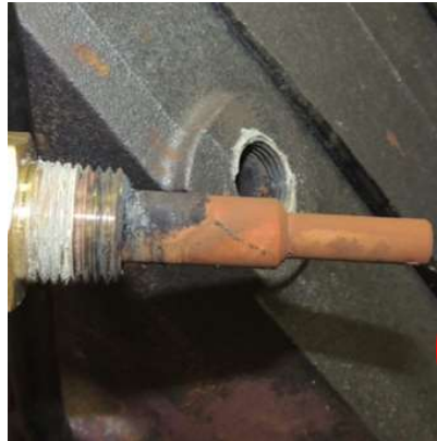
LWCO Probe fouled
